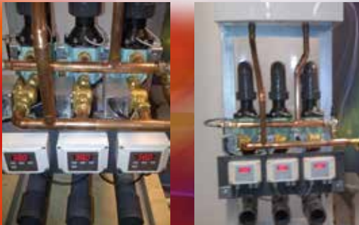
A typical multi-tub boiler heating installation
